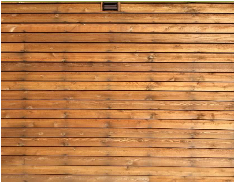
2-year-old wall face with bleeding face nails
